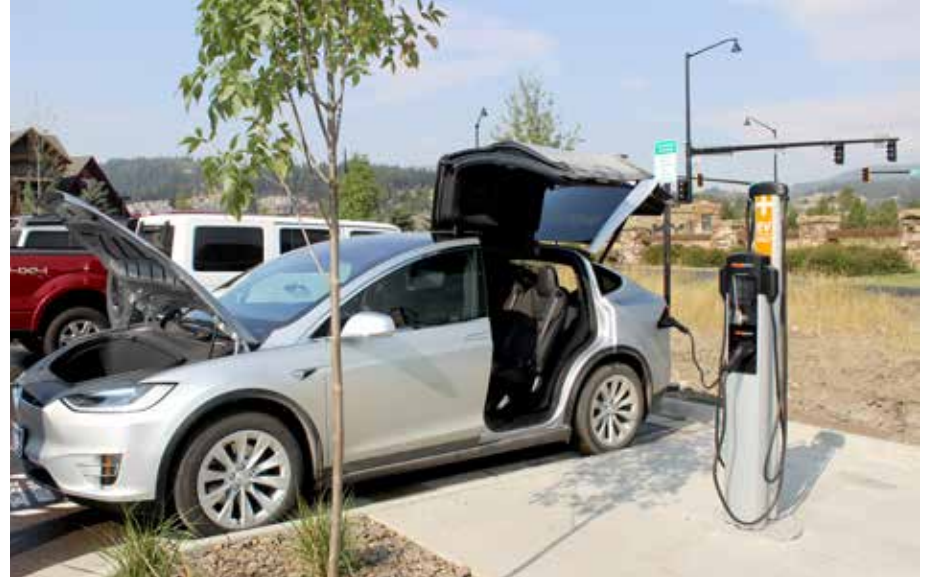
Big Sky's first public electrical vehicle charging stations are now ready for use. The two stations are located in Town Center behind the Big Sky Exploration Center and can charge up to four vehicles at a time. PHOTO BY BAY STEPHENS
