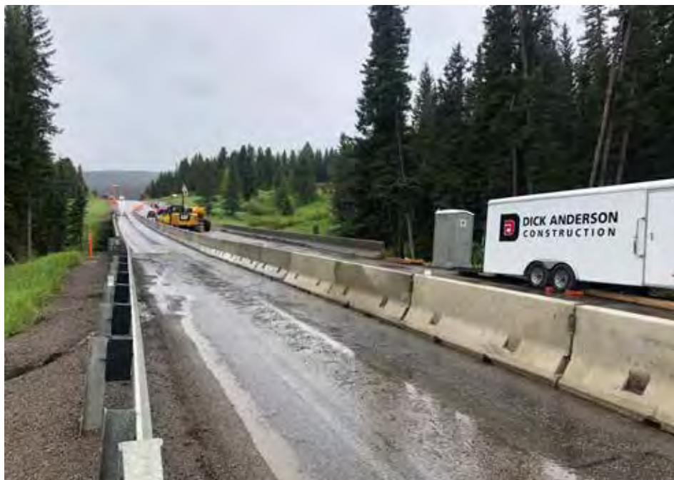
Construction underway on the Middle Fork bridge, located on Highway 64 near the intersection with Little Coyote Road. PHOTO BY BELLA BUTLER
