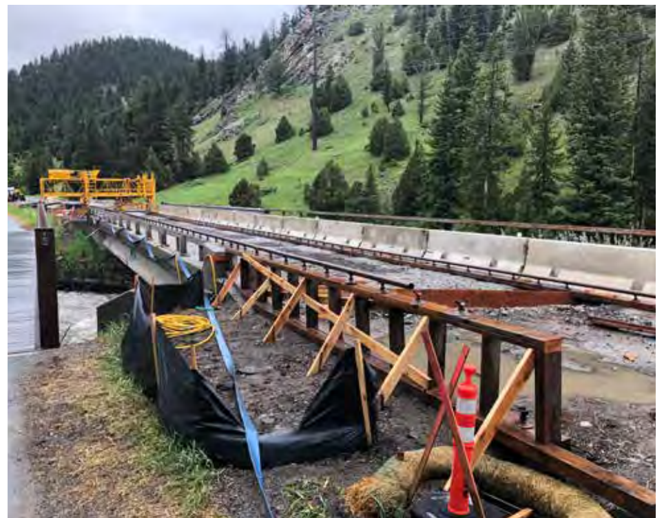
Construction underway on the West Fork bridge, located on Highway 64 near the Conoco and Big Sky Chamber of Commerce. PHOTO BY BRANDON WALKER
