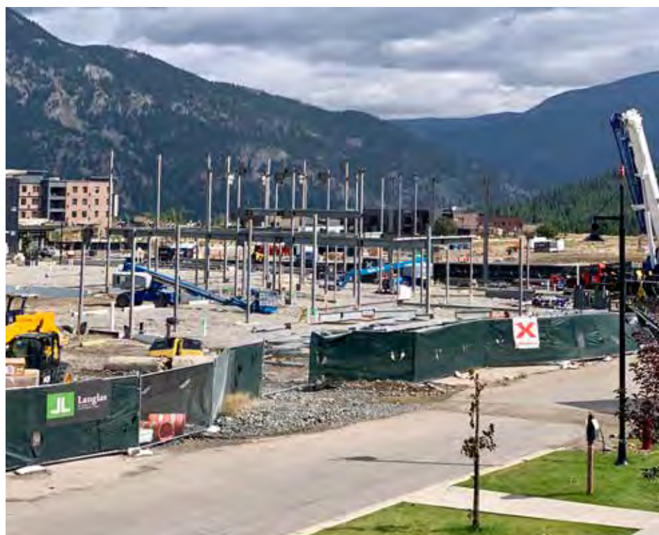
The new BASE community center is making fast progress—this month underground plumbing and foundation were completed. PHOTO BY TUCKER HARRIS
